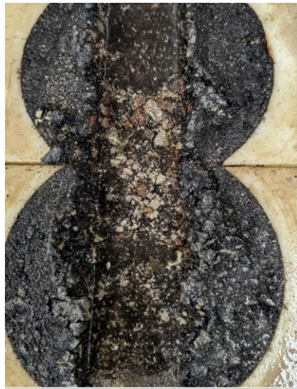
Figure 3.1. Mix Experiencing Severe Stripping and Rutting
