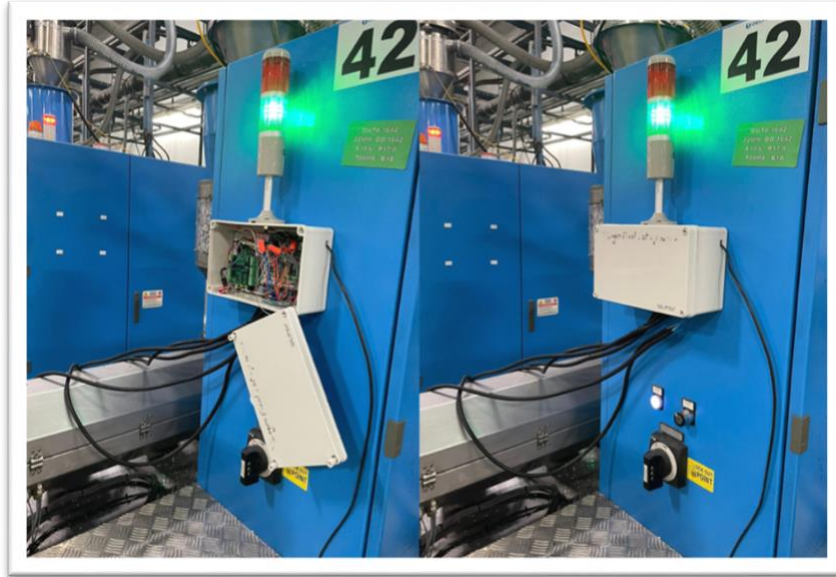
Figure 4.3 Temperature Sensor Module Installed on Equipment #42
