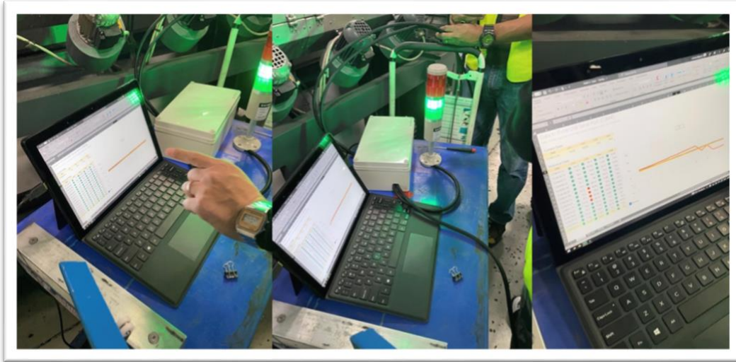
Figure 4.2 Temperature Sensor Module Tested On-Site
