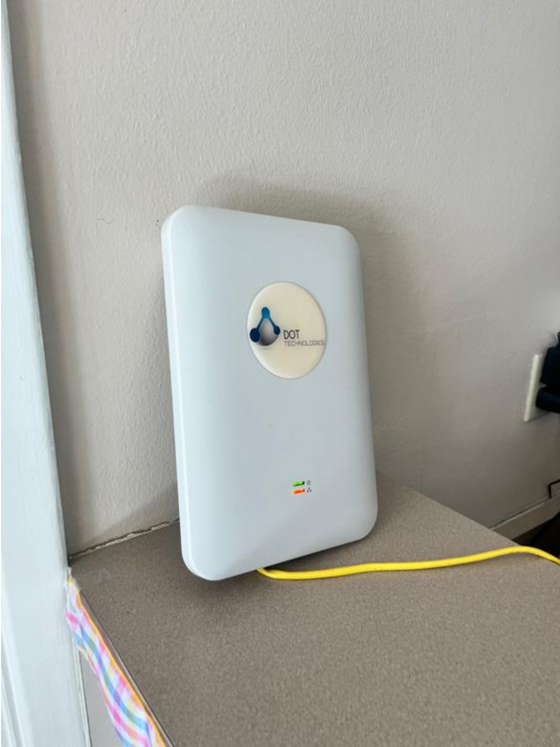
Illustration 4.6: Newly Installed Cambium Network Access Point
