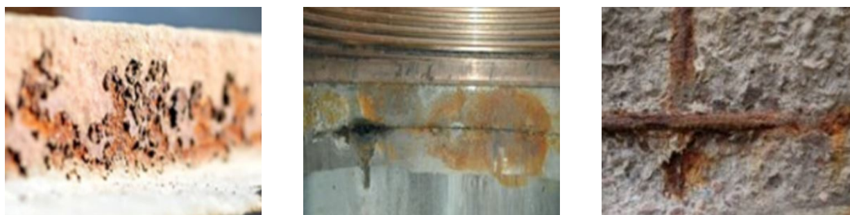
(a) Pitting Corrosion
