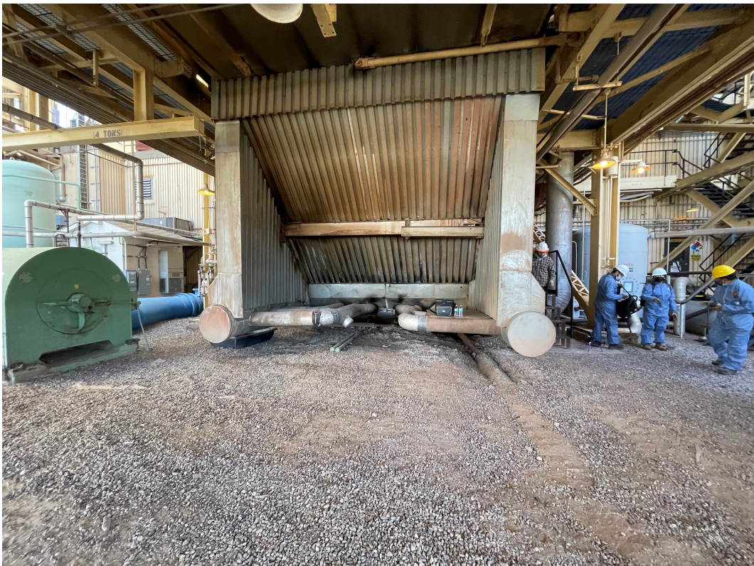
Figure 7.8: EPE Rio Grande - Power Unit - Outside of Boiler Furnace
