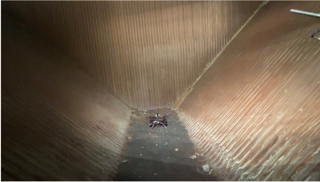
Figure 7.9: EPE Rio Grande - Power Unit - Inside of Boiler Furnace
