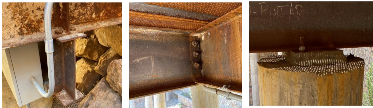
Figure 8. Photo. Steel beam to girder bolted connection(left), beam to beam bolted connections (center), and haunch at steel girder and reinforced concrete column connection (right)
