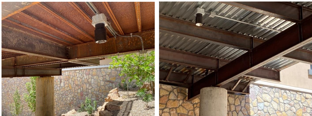
Figure 7. Steel channel planks (left) and concrete slab on metal sheet for decking (right)
