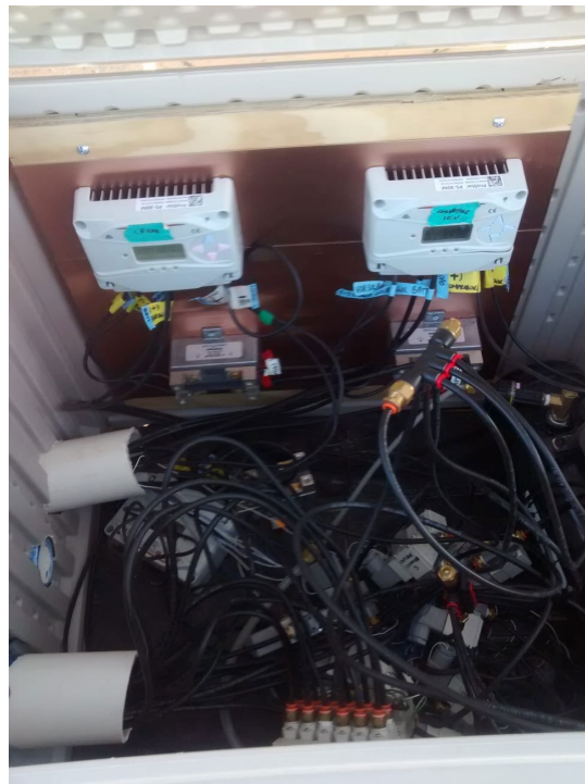
Figure 2.10 Controllers, polyphasers and two port valves interconnected to control the airflow of the automated flux chambers.
