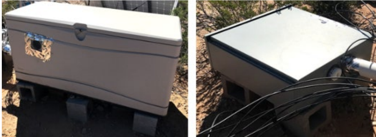
Figure 2.13 Weather resistant enclosures for electronic equipment at The Jornada LTER
